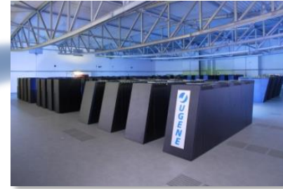
Supercomputer & Data center
